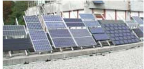
Figure 1: View of the LEEE-TISO test facility with the 14 modules under test in cycle 8.
