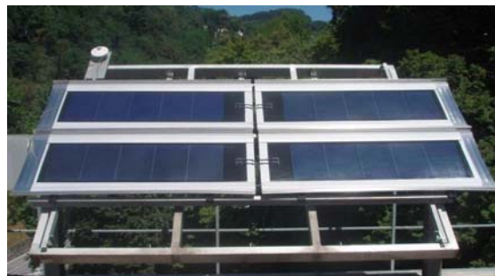
Fig.1: Outdoor installation for monitoring of Riverclack ® Elios Deck PV modules during degradation.
